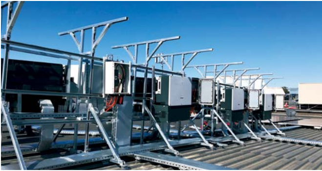
1 MW PV Plant Australia
