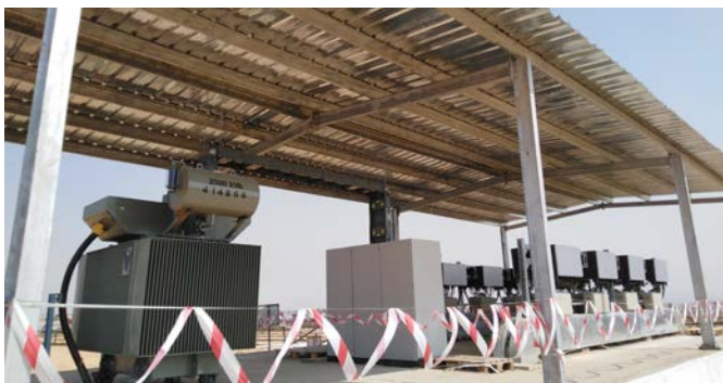
10MW PV Plant Pakistan
