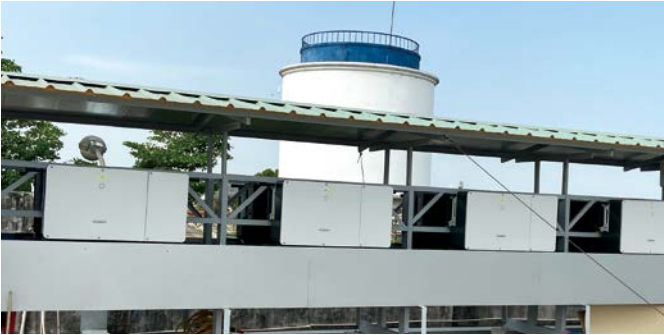
1 MW PV Plant Vietnam
