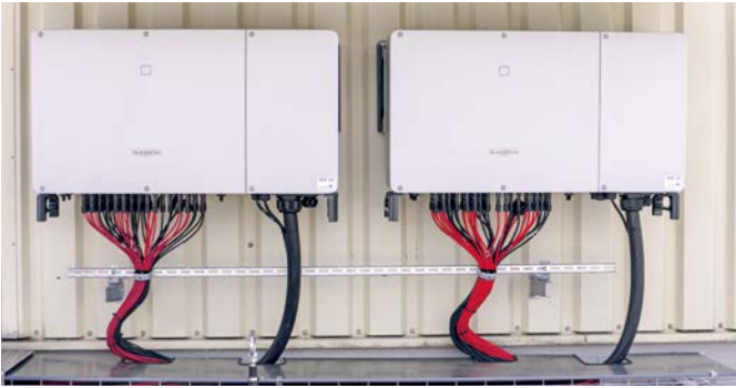
550kW PV Plant Germany
