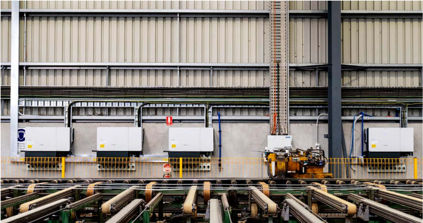
520 kW PV Plant Australia
