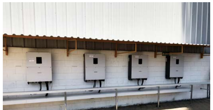
6.5 MW PV Plant Spain
