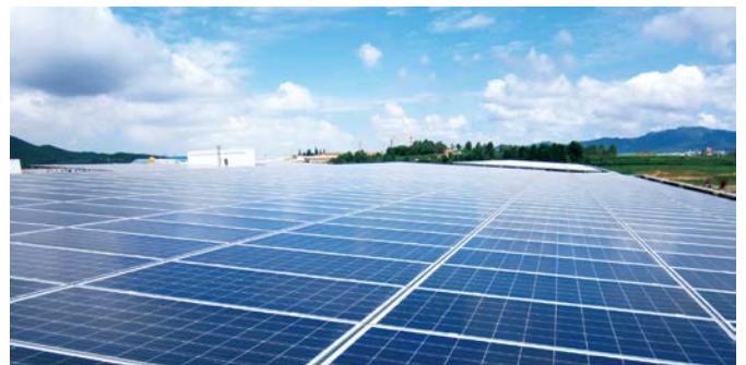
1.4 MW PV Plant Vietnam
