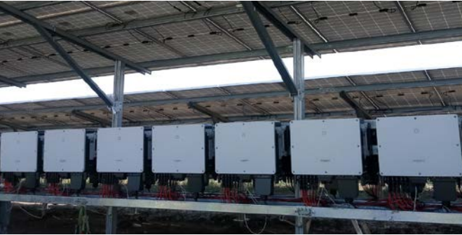
950kW PV Plant Korea
